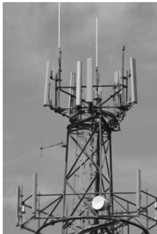
One of 'The Mobile Phone Company's masts, near Sometown, Wessex.
